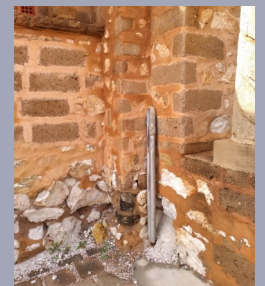
Fretting external stone-work
