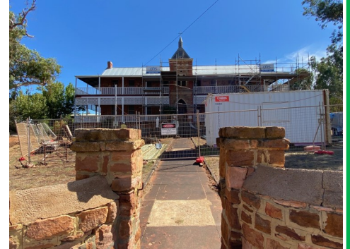
Above: Convent in Northampton still to be repaired fully
